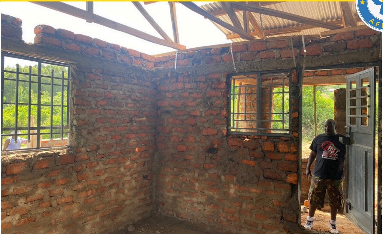
Above: Jeff, one of our Kenyan board members, inspects the front door installation.
